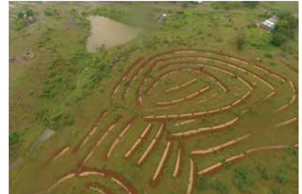
DEEP CONTINUOUS CONTOUR TRENCH (DCCT) – The depth of DCCT goes up to 1 meter. These are generally constructed in areas with low slope and less evaporation.
