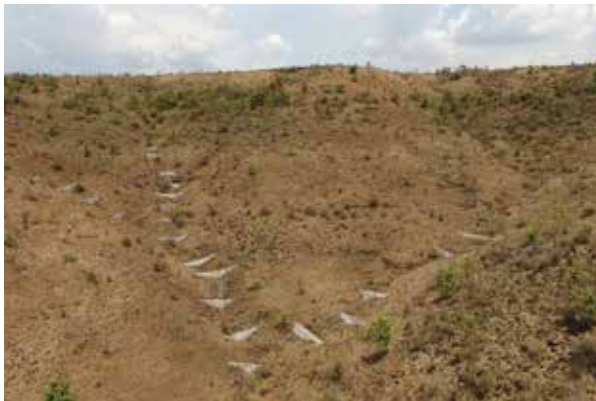
LOOSE BOULDER STRUCTURES (LBS) – These are small check-dams constructed by stacking loose boulders in drainages with less flow of water. They arrest the silt and increase the water percolation.
