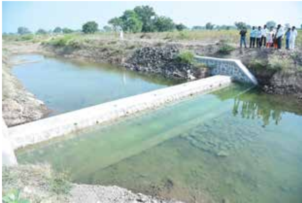
CEMENT NALA BUND (CNB) – These are concrete structures built in a stream or small river to harvest water.
