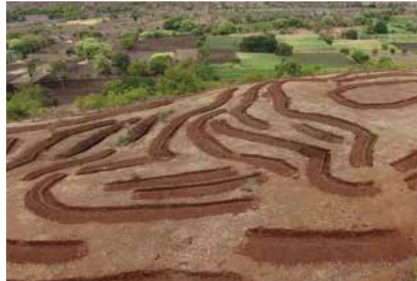
CONTINUOUS CONTOUR TRENCH (CCT) – These are small trenches built along the contour lines in the common land to trap and percolate more rainwater.
