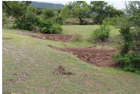
GULLY PLUG (GP) – These are LBS and serve the same purpose, however these are constructed with some waste materials.
